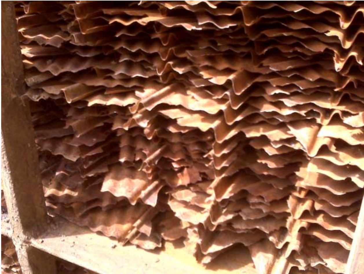
TWO LAYER COLD END DAMAGE
